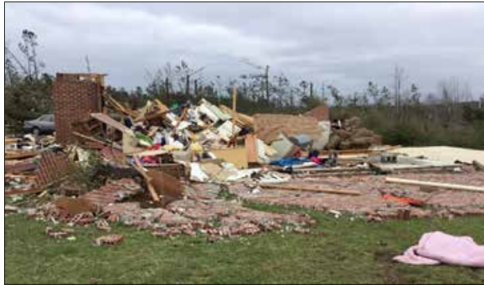
One of the homes destroyed by a category EF-4 tornado in Lee County on March 3, 2019.
