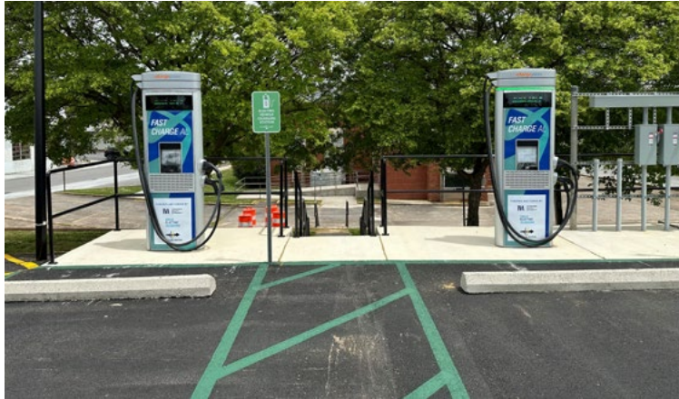
The new fast charging station at 214 Chestnut Street NW helps both local electric vehicle drivers and those traveling through our region. Located within walking distance of restaurants and downtown shopping, the new station provides convenience and supports local businesses.
